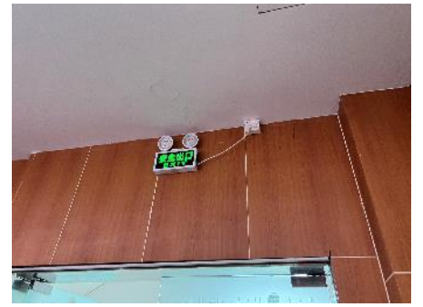
Emergency light/Exit sign
